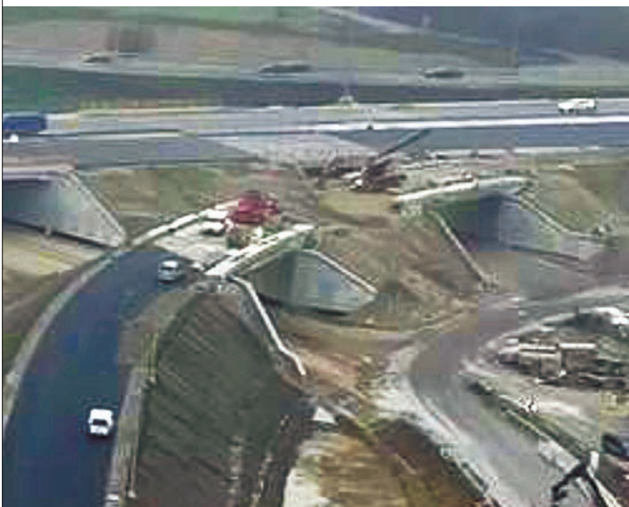
Obr. 6 Most na D1 a kolektorovom páse ponad križovatkové vetvy Fig. 6 Bridge on the D1 and collector road spanning the junction branches
