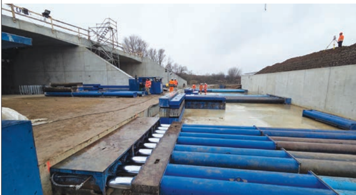
Obr. 5 Fáza zatláčania konštrukcie do telesa násypu Fig. 5 The construction stage of pushing the structure into the embankment body
