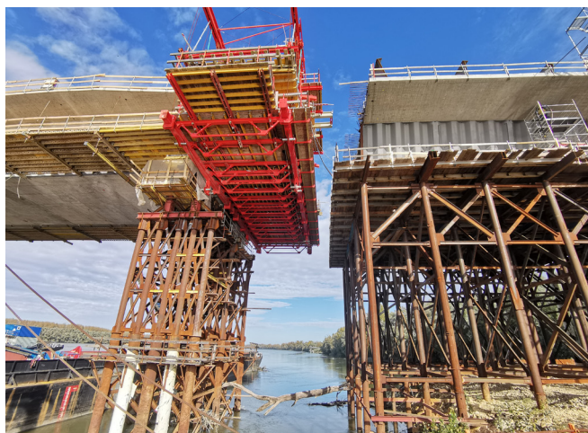
Fig 12: SJ2 temporary support and scaffolding below the segments P24-P20, prior to the assembly of the closure segment
