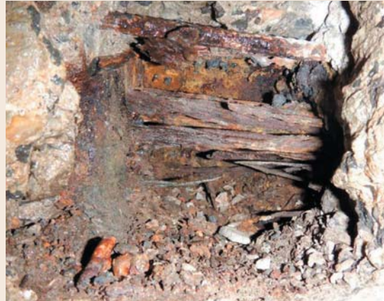
Fig. 4 Corrosion of prestressing steel
