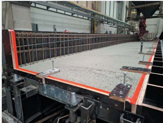
Fig. 2 Manufacturing of a precast grandstand unit: casting into the mould with installed reinforcement (LC35/38 D1,8; flow class F5)
