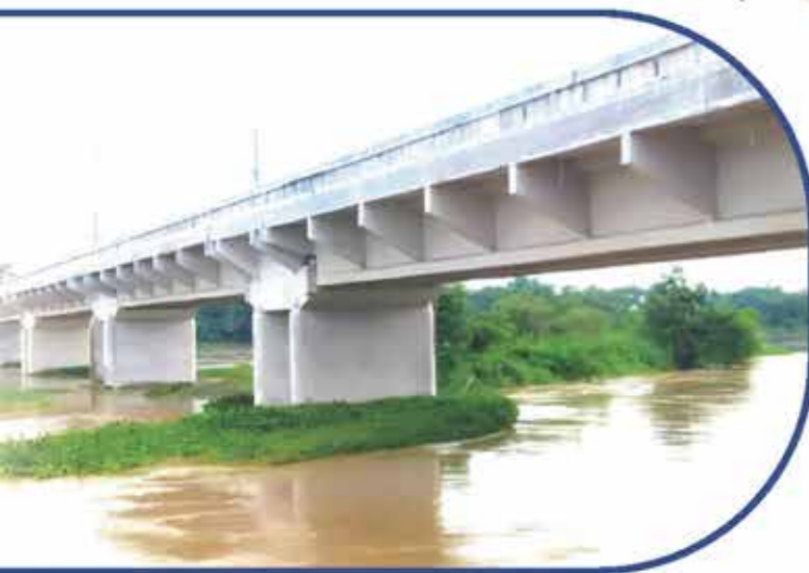
Structural Retrofitting of Dilapidated Bridge on NH14 over River Kangsabati, West Medinipur, West Bengal
