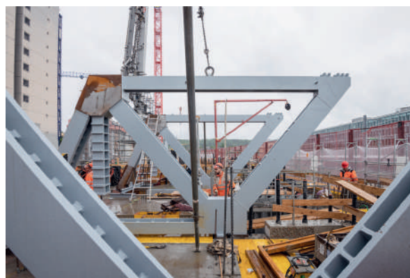
Fig. 5 Stahlfachwerke der Kernabfangung. Steel trusses as inserts in concrete core walls. (© Beat Bühler)
